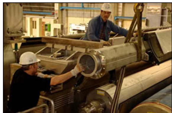
The VIB SteamTech profiler being lowered by crane, and connected to the retraction unit and the utility pipes.
