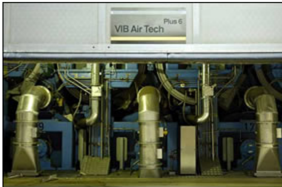
A perfectly integrated VIB AirTech Plus 6 -spray in the drying unit.
